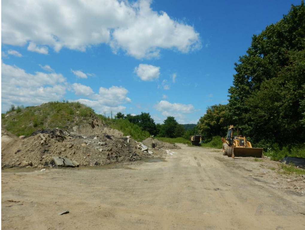
Photo 7. The County of Westchester has long used this area in the central-southern portion of the Project for dumping. View looking north.
